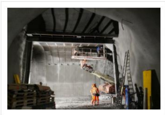
Finalising work at the breakout adit junction with the main running tunnel
