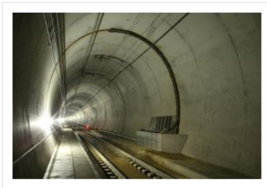
Temporary sedimentation tanks in the east running tunnel ahead of the permanent works
