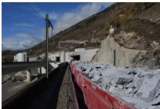
Access provided via the closed east tube from the Raron portal of the railway
